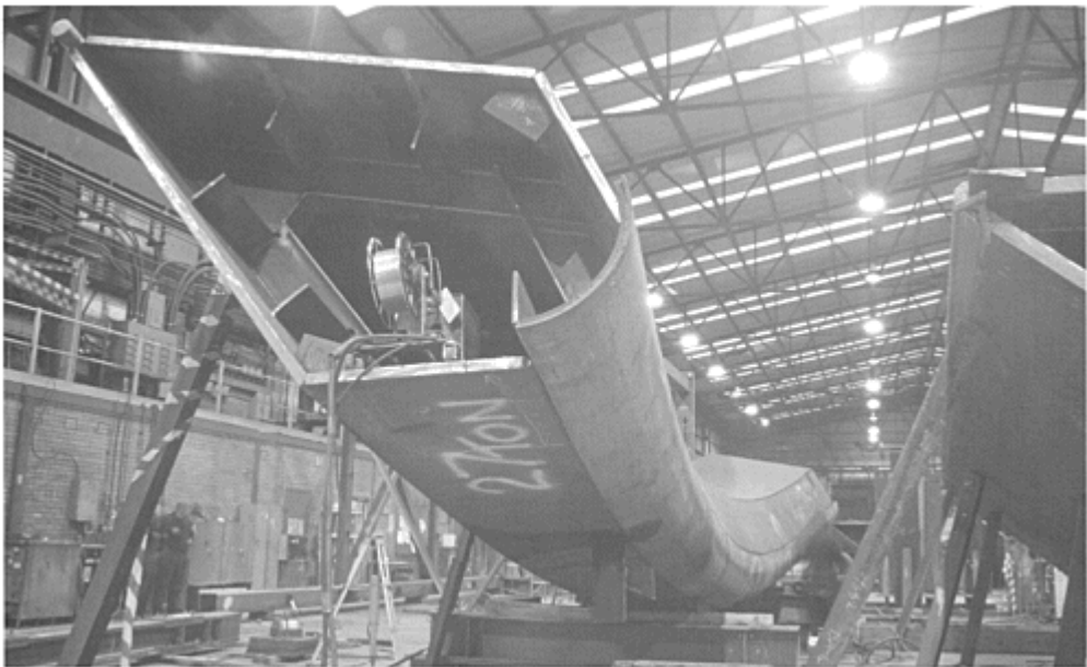
13.11 Gateshead Millennium Bridge, 2001: section of the arch structure in the fabrication works Guy Hearn, photo used with kind permission from Gateshead Council
