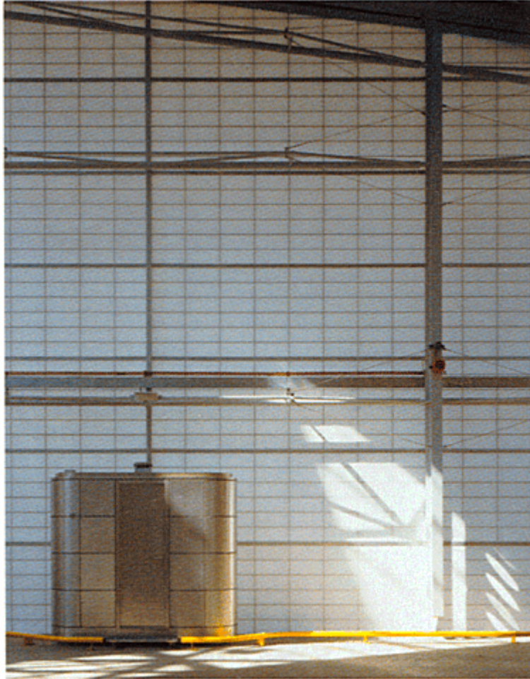
13.14 The translucent composite cladding on the south elevation of Stratford Market depot provides a glowing light like the Japanese shogi
