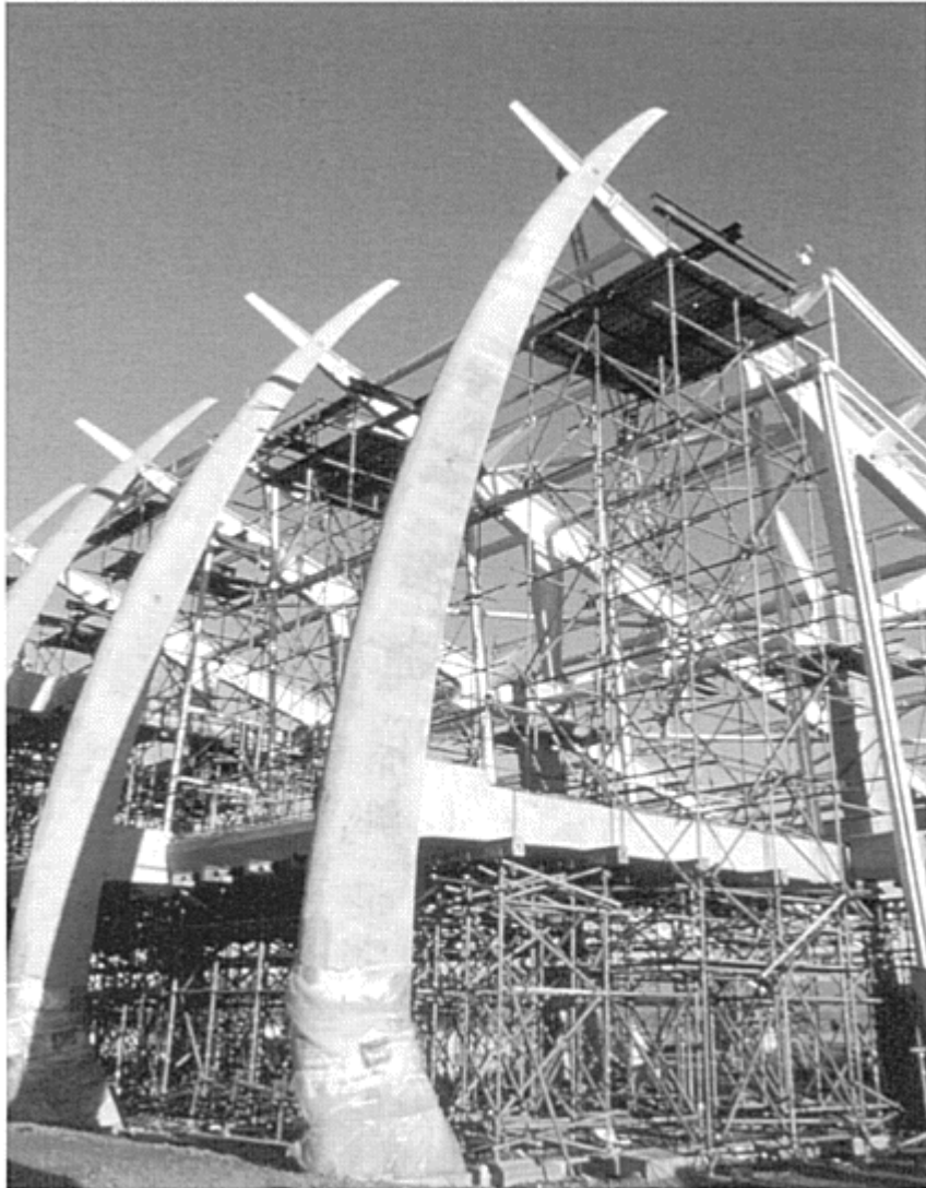
5.9 Greenock Waterfront Leisure Complex, 1996: concrete ‘tusks’ being erected (architect: FaulknerBrown) needing only simple tools to extract it from the land. The building process is also fairly straightforward and the construction material is totally recyclable.
